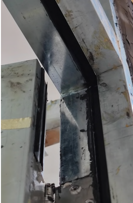
Photo 18 - The top left corner of doorset after medium temperature test
