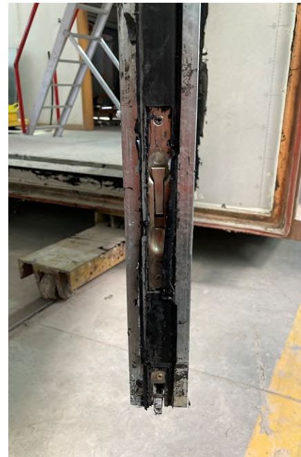
Photo 10 - The position of flush bolt after medium temperature test
