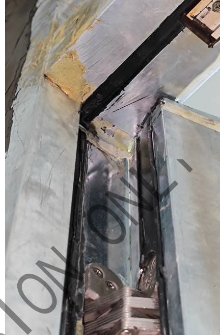
Photo 19 - The top right corner of doorset after medium temperature test
