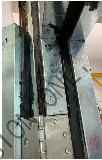
Photo 4 - The top right corner of doorset after medium temperature test
