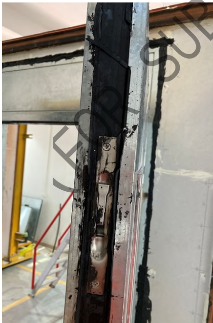
Photo 9 - The position of flush bolt after medium temperature test
