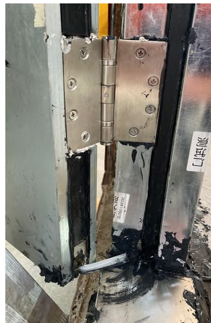
Photo 6 - The bottom right corner of doorset after medium temperature test
