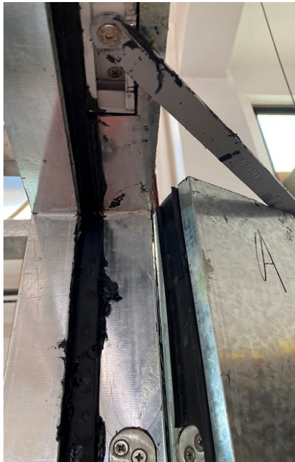
Photo 3 - The top left corner of doorset after medium temperature test
