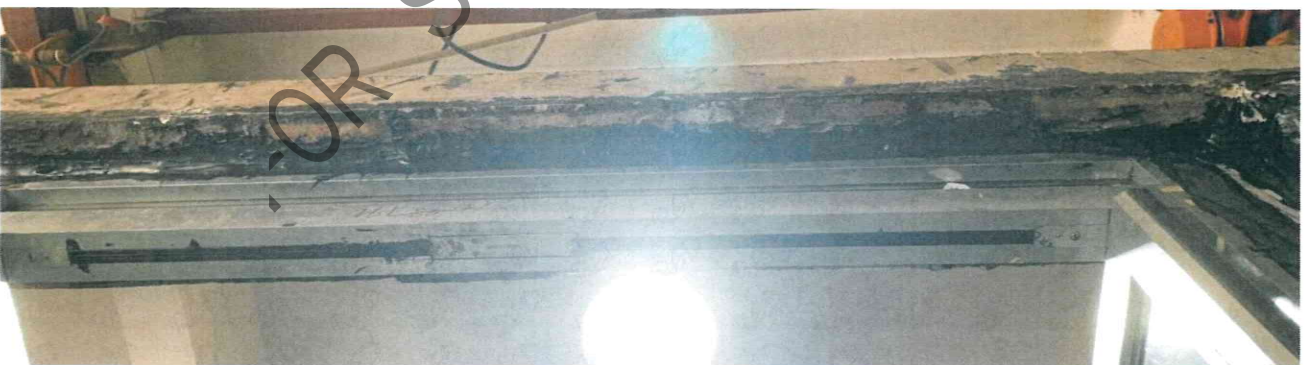
Photo 4: Fire seal & smoke seal arrangements at the head of door frame
