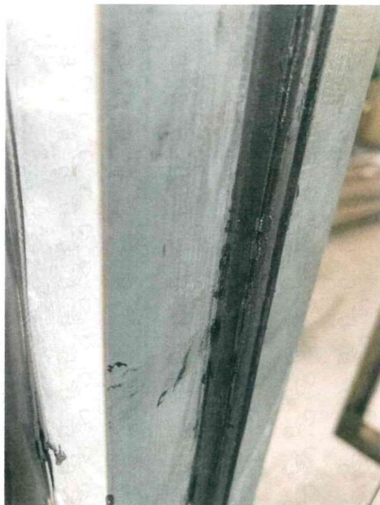
Photo 5: No smoke seal arrangements at the door frame vertical jamb
