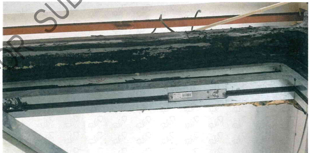
Photo 4: Fire & smoke seal arrangements at the head of door frame
