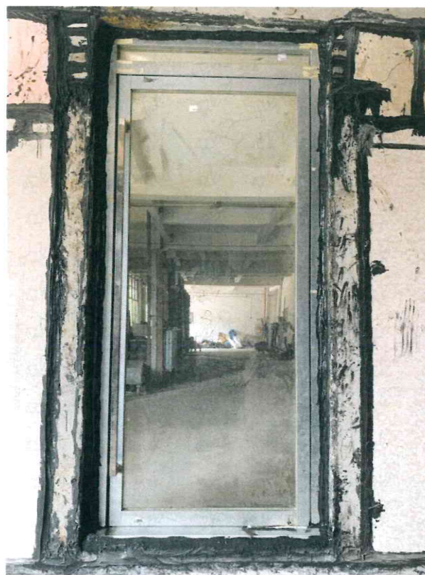
Photo 2: Exposed face of Doorset after the test.
