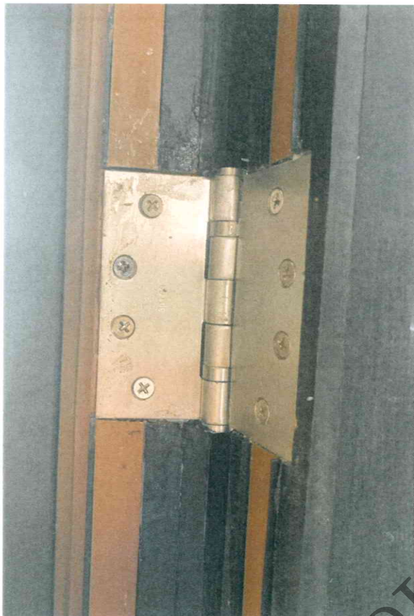
Photo 9: Interruption of the fire and smoke seal at the hinges position
