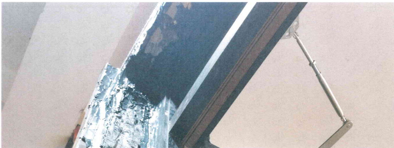
Photo 7: Fire and smoke seal arrangement on the head of the door frame
