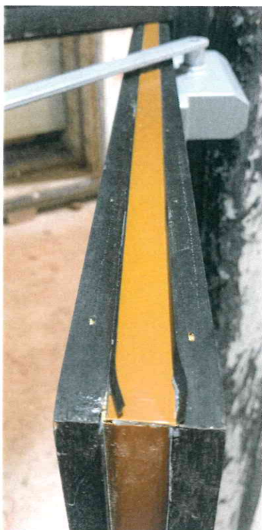
Photo 7: Fire and smoke seal at the top edge of the door leaf
