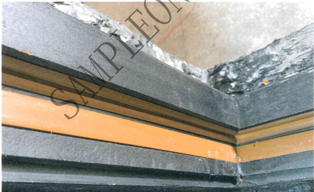
Photo 6: Fire and smoke seal at the vertical jamb of door frame
